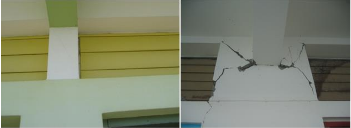
Figure 1: Diagonal cracks in the short columns
