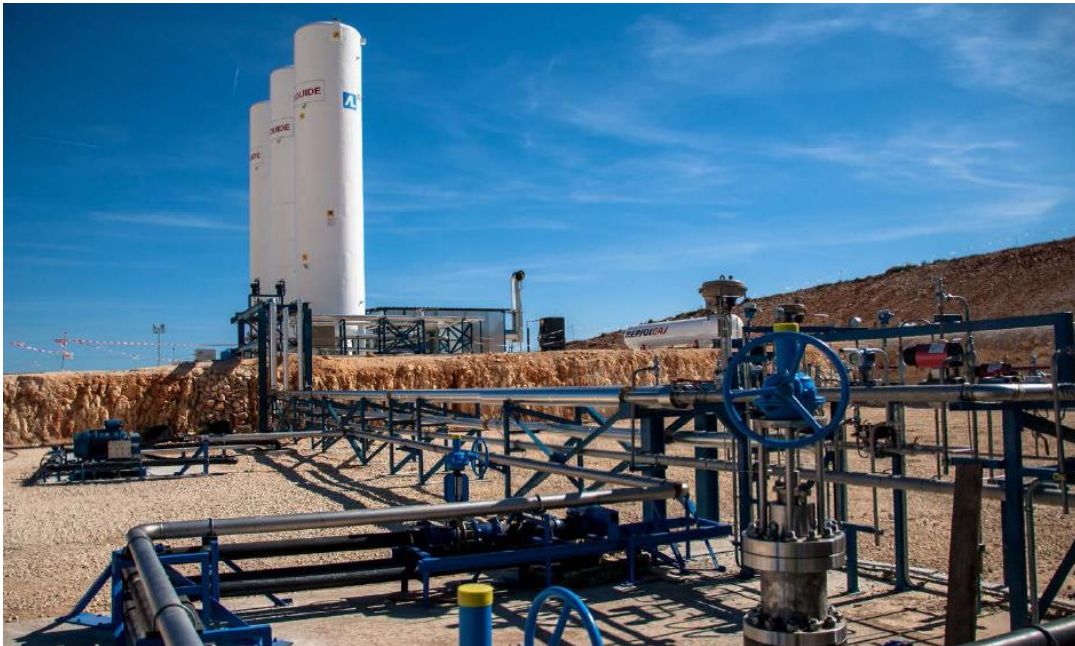
Figure 2: The Hontomin Pilot site: injection infrastructure and CO 2 tanks
